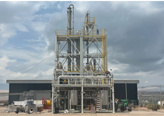
Figure 1: NCCC UNOGAS commercial pilot plant prior to installation.
